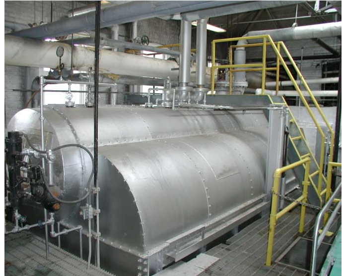
1957 Keeler Boiler rated at 20,000 lbs/hr
